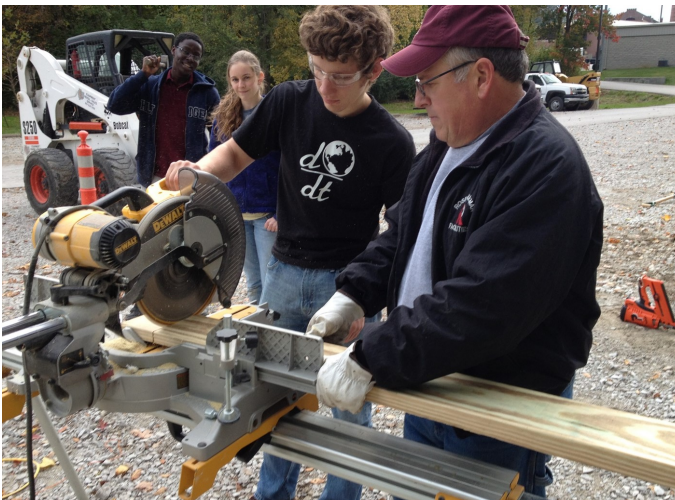
HERE freshmen partnered with facilities staff to construct a passive solar greenhouse on campus.
